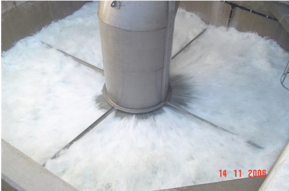
Photograph 4 DV discharging radially into chamber to dissipate energy
